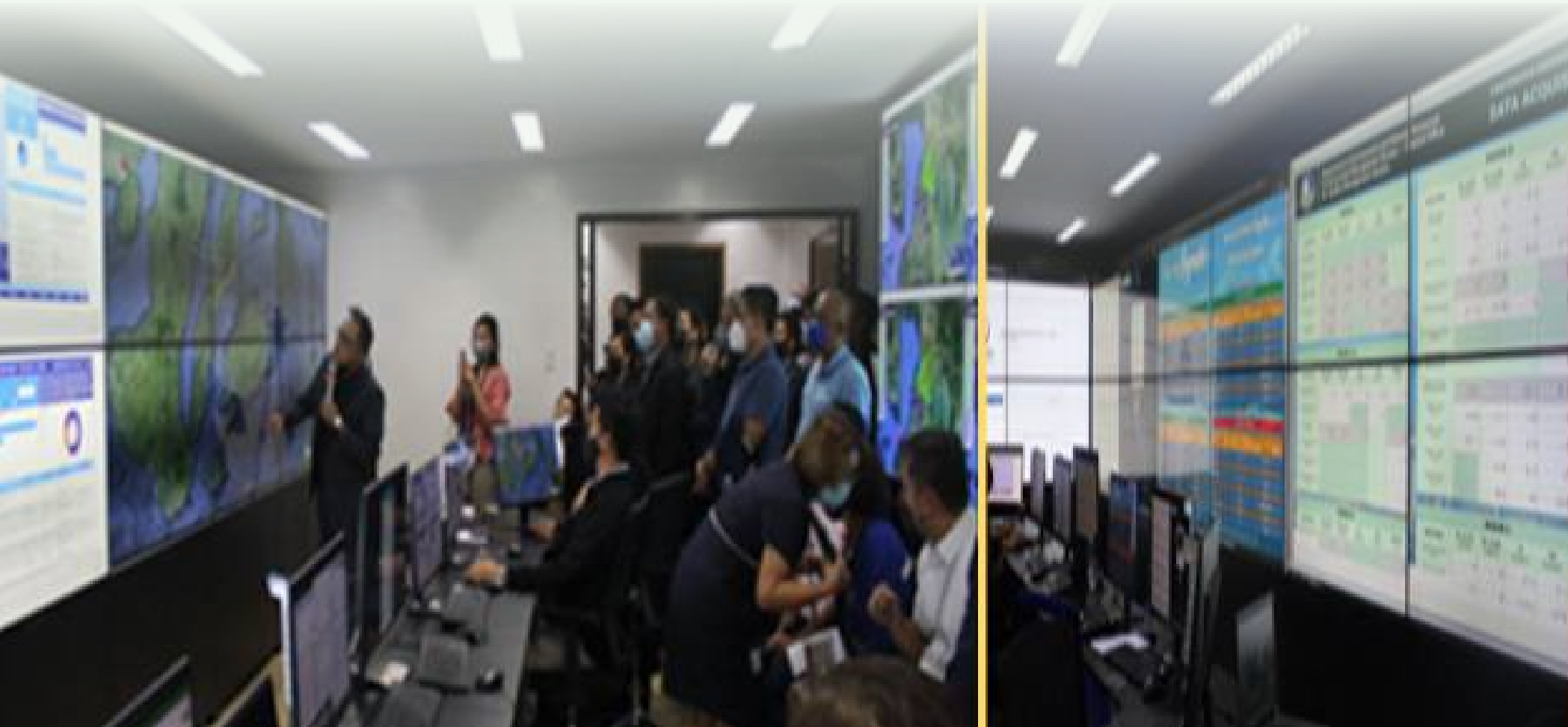
EMB Data Center
