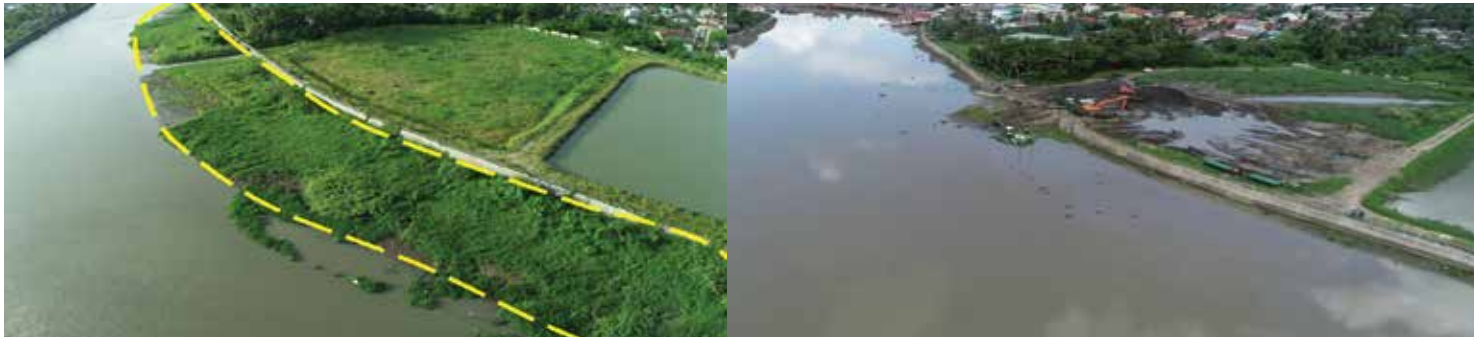
Before and after the Phase I dredging in Brgy. San Roque, Camaligan, Camarines Sur
