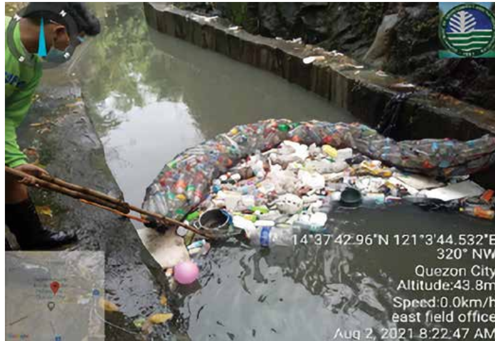
Installation of floating trash trap in Buaya Creek in Brgy. Quirino 3A, Diliman, Quezon City
