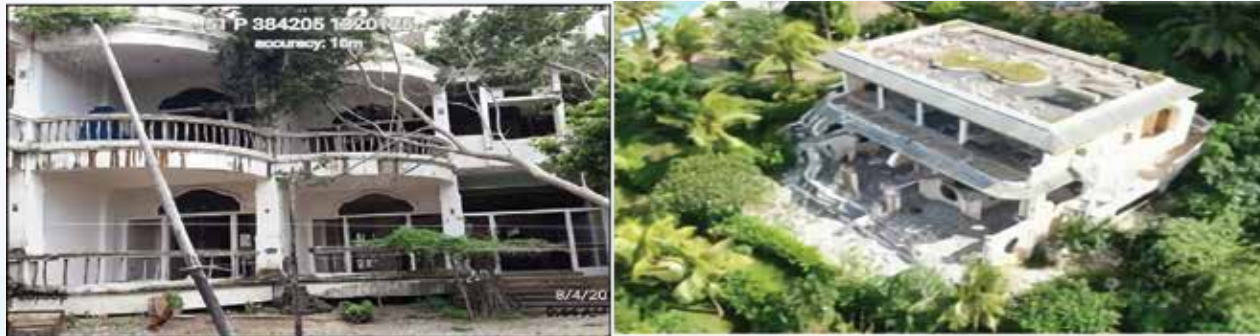
Demolition of Lasatin Residential House at Diniwid Area and Monaco Suites de Boracay (L to R)
