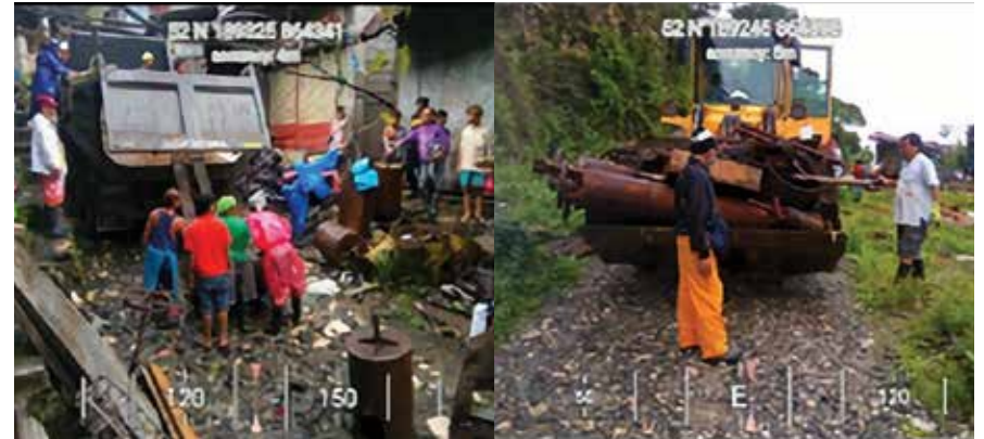
Transfer and hauling of mineral processing plants from Mt. Diwata to Mabatás Mineral Processing Zone, Upper Ulip, Monkayo, Davao de Oro
