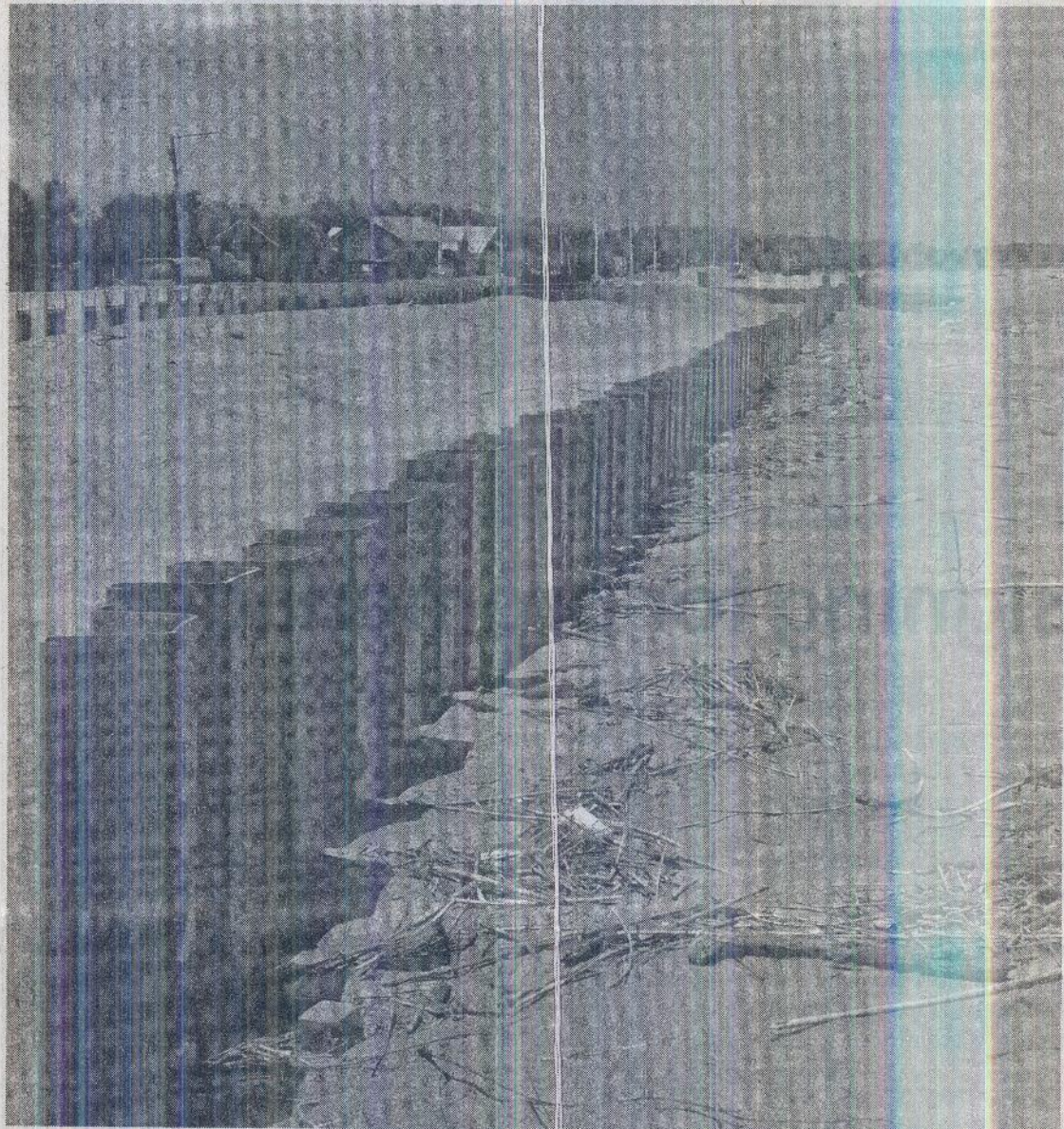
NOT GOOD? Sheet piles, which mark the extent of the Lingayen-Binmaley seawall, configure the shoreline of Lingayen Gulf as construction of the seawall continues despite the protests from local fishermen groups. PHOTO BY GABRIEL CARDINOZA
