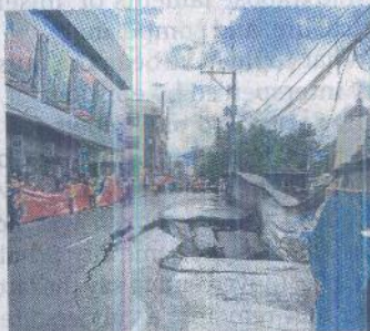
AFTERMATH A section of Legaspi Street in Cebu City caves in on Wednesday amid heavy rains and floods this week. —PHOTO COURTESY OF CEBU HILIG UG MOTO
