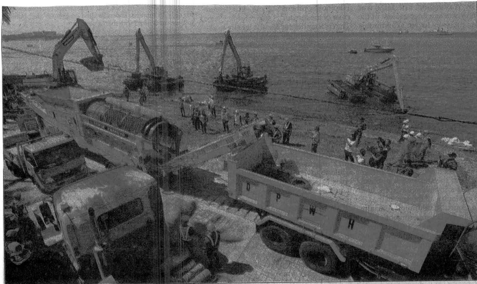
Department of Public Works and Highways personnel operate amphibious excavators to remove silt from Manila Bay's shoreline yesterday.
