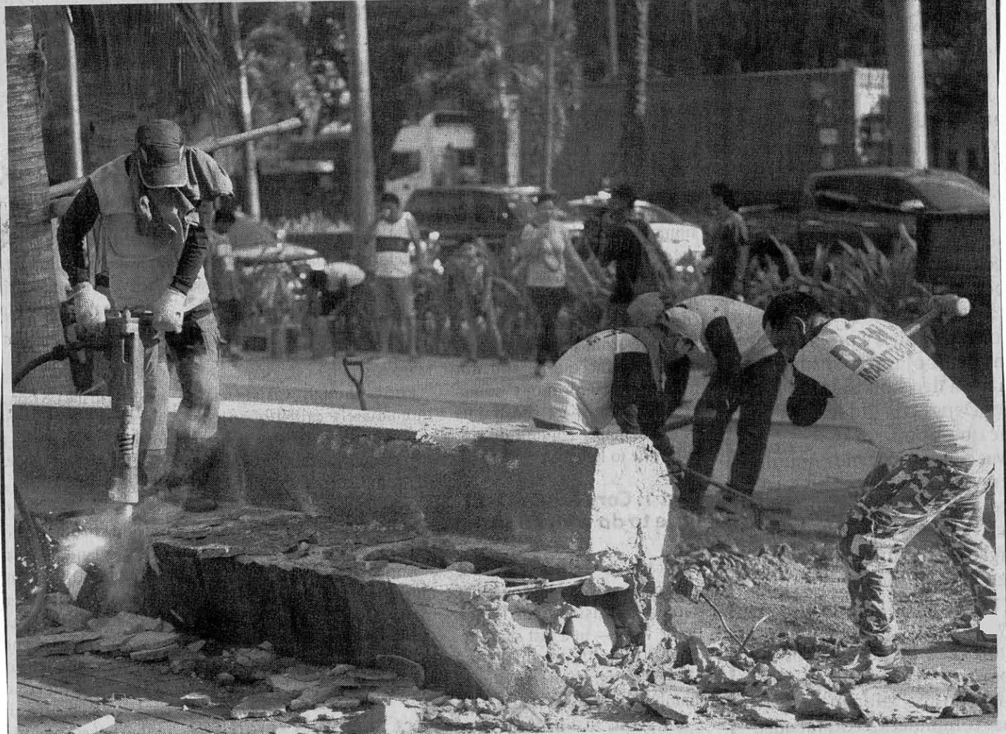
OFF WITH THE BENCHES Workers demolish benches along Baywalk in Manila as the rehabilitation of Manila Bay continues. PHOTO BY RUSSELL PALMA
