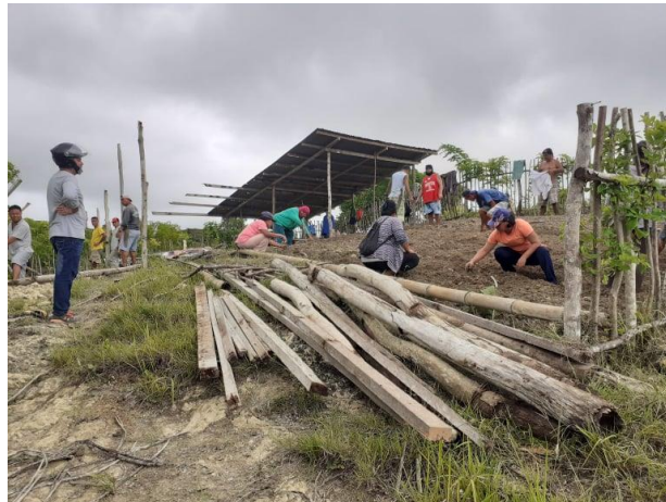
BAYANIHAN. Construction of MRF by barangay councilors and other officials and volunteers of Barangay Basac in Larena, Siquijor using only indigenous materials and madre de cacao as fence trees as as fence. (rac/PIA-Siquijor with photo from MJ Banglos/Zero Waste Foundation)
