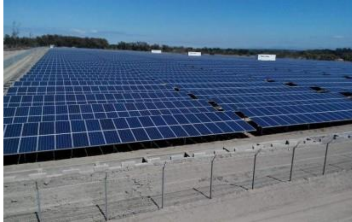
Solar energy farm in Currimaos, Ilocos Norte (PNA photo by Leilanie G. Adriano)
