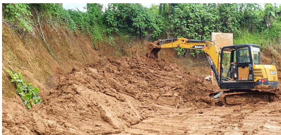
A personnel from the Department of Public Works and Highways continues removing the mud deposits caused by soil erosion in Lakeview Transitional Shelter Site (TSS) in Barangay Boganga on Friday evening. (TFBM Field Office)
