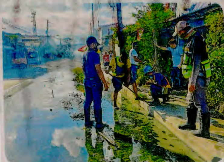
In Zamboanga City, LGU representatives address flooding challenges by declogging, fixing and cleaning drainage canals and pipes.
