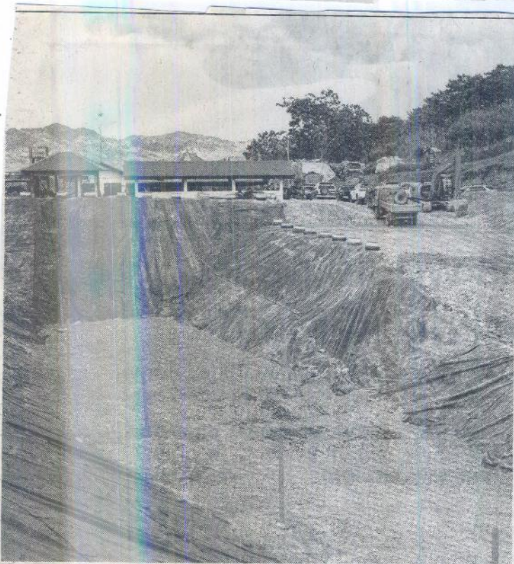
PARTNERSHIP PRODUCT The town of Kasibu in Nueva Vizcaya, jointly with the Didipio Mine, constructs a modern landfill to improve management of waste disposal in 30 villages of the municipality. CONTRIBUTED PHOTO
