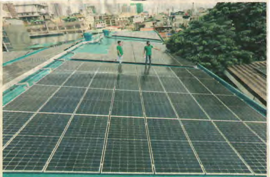
Shown in photo is the solar rooftop installation at Mary Johnston Hospital in Manila designed to produce over 10 million kWh of solar-generated electricity for 25 years. (Noel Pabalate)
