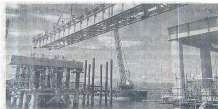
■ AG&P's liquefied natural gas (LNG) terminal under construction in Batangas. AG&P PHOTO
