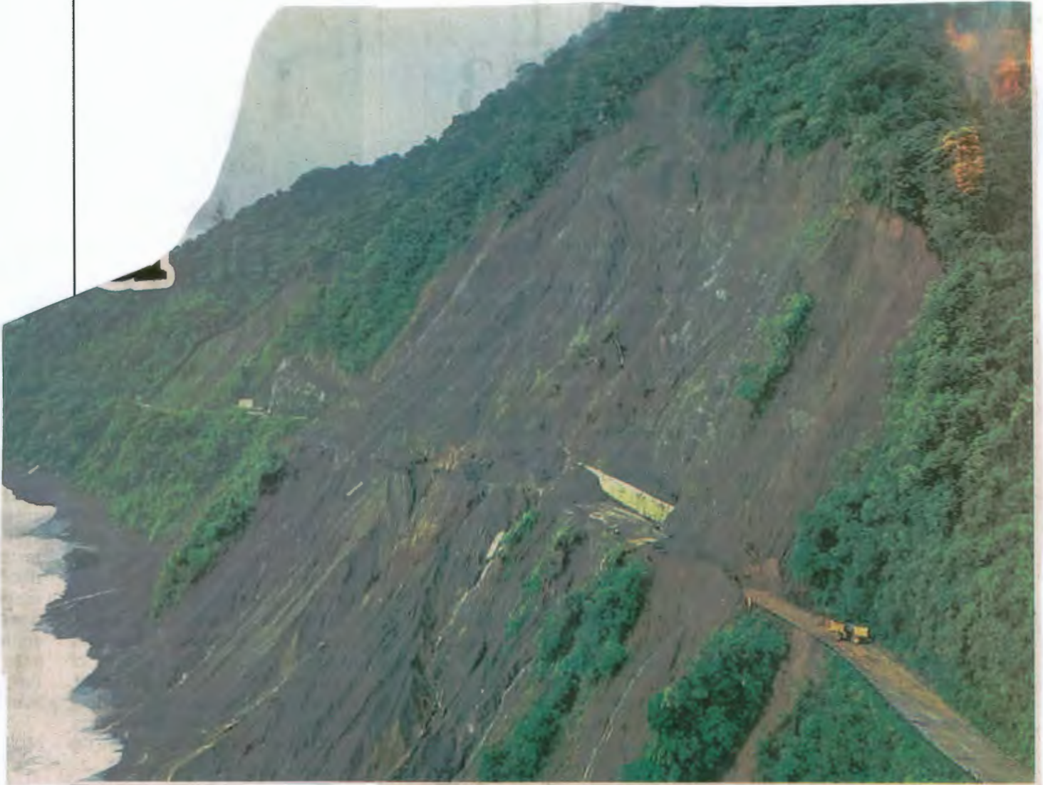
SHUT DOWN – The Manila North Road in Barangay Pancian, Pagudpud, Ilocos Norte is closed to traffic on Friday, Oct. 21, 2022, after a landslide. (DPWH photo)
