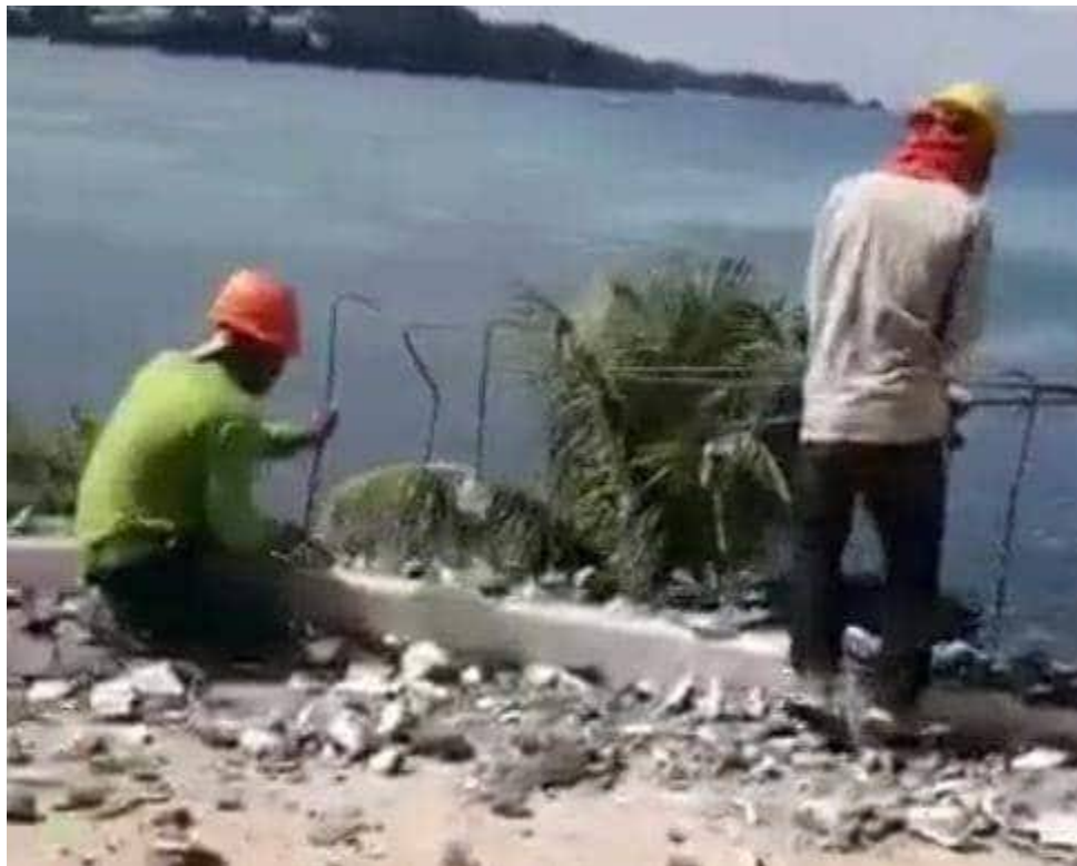
A still from a video of the demolition of a portion of the Monaco Suites de Boracay in Boracay Island. (Courtesy of Boracay Informer/Manila Bulletin)
