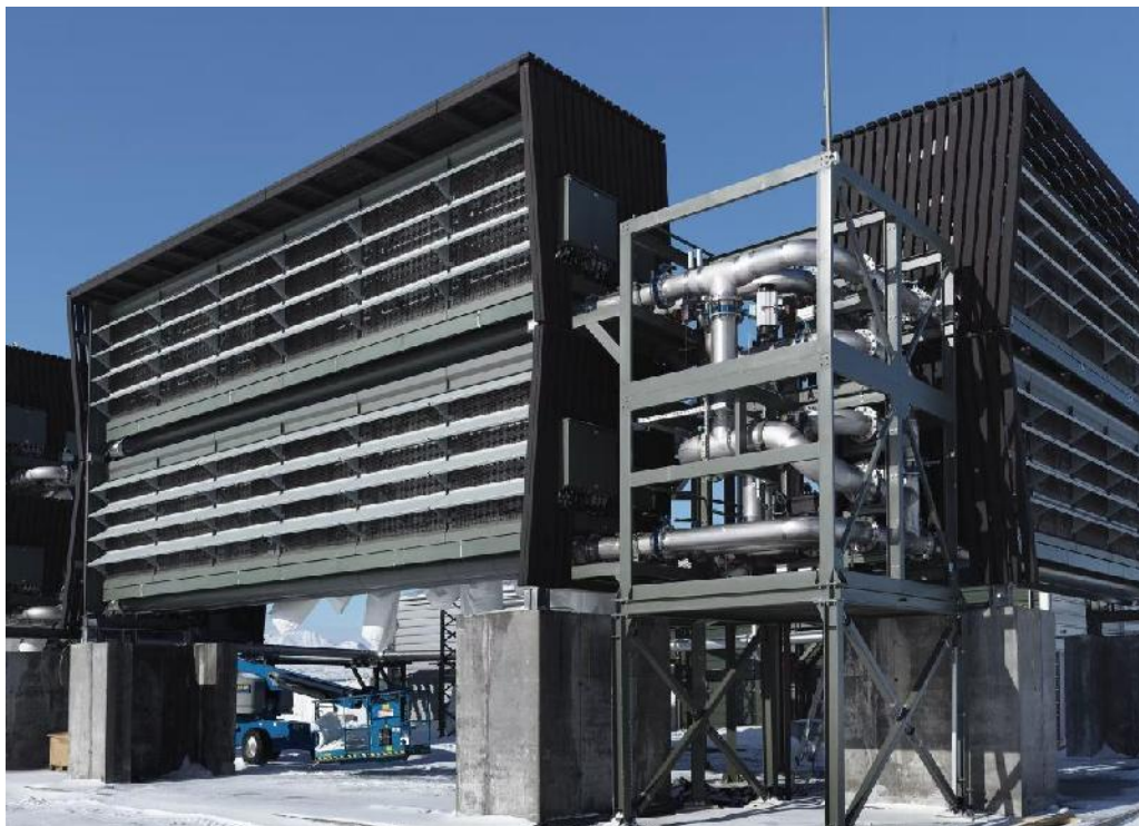
World largest direct air capture plant in Iceland, built by Swiss firm Climeworks. Image: Climeworks.
