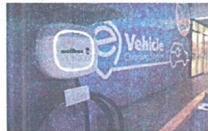
Two Wallbox Pulsar Plus 7.4KW AC chargers with Type 2 connectors are deployed at each of four SM Supermall locations.
