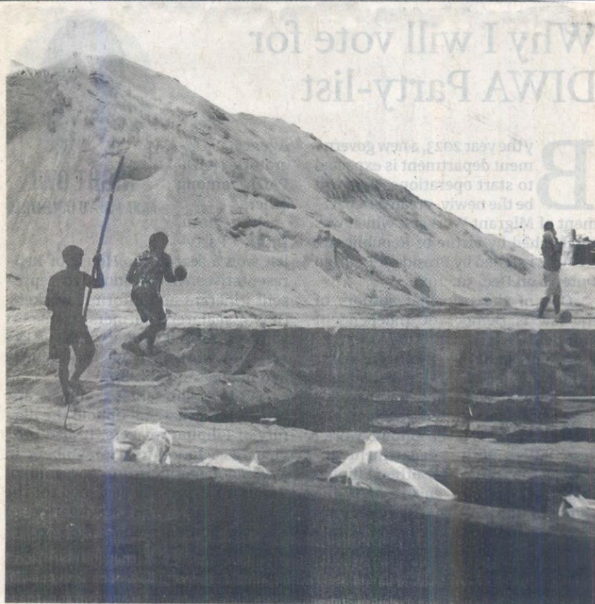
BEAUTIFICATION PROJECT – A huge mound of sand is delivered by a barge on the banks of Manila Bay on Roxas Boulevard in Malate, Manila, on Tuesday, March 8, 2022, as the beautification of the Manila Baywalk Dolomite Beach continues. (Manny Llanes)
