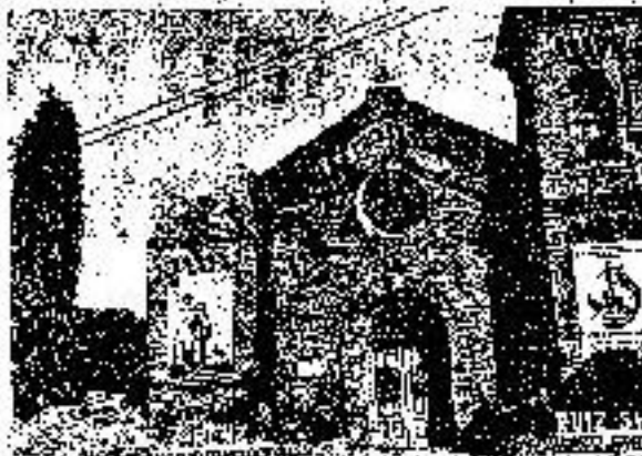
Although the stone church in Abra, also known as the St. Catherine Church, suffered big cracks, it is considered a national cultural treasure, being the oldest and largest in the Cordillera region.
