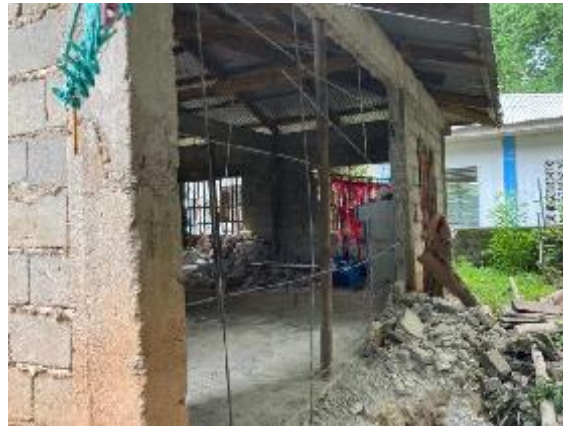
A damaged house in Abra (Daniza Fernandez / INQUIRER.net)
