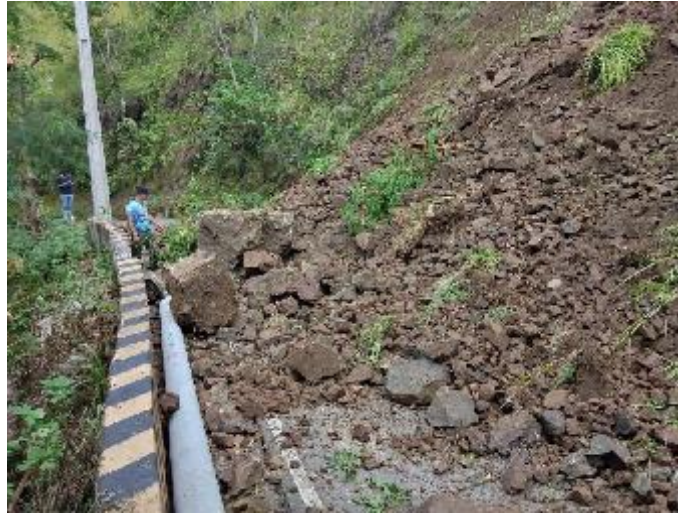
Landslide on portion of Andres Acop Cosalan Road in Poblacion, Bokod, Benguet on July 27, 2022 after Abra quake. Photo: PROCOR PIO
