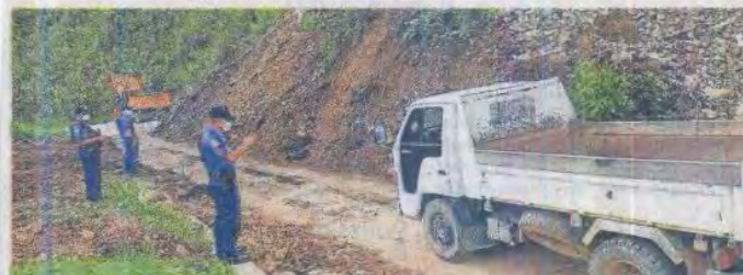
REOPENED Policemen in Banaue, Ifugao province, on Tuesday assist motorists through a reopened section of the Banaue-Hungduan-Benguet boundary road. A landslide blocked the road during heavy rain on July 7. —PHOTO COURTESY OF IFUGAO POLICE
