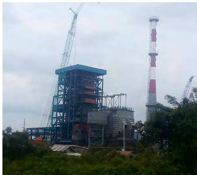
DMCI Power Corp. coal plant under construction in Masbate in 2019. This should have been the last coal plant built in the Philippines, but it won't be. Photo by the author
