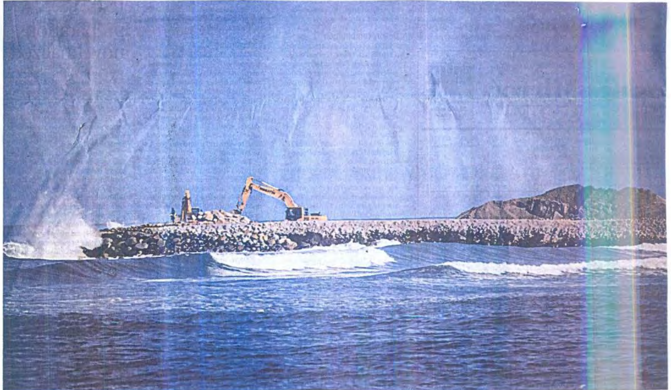
'NO EXPENSE?' A massive dredging operation continues near the mouth of a river facing the West Philippine Sea in Cabangan, Zambales, to help mitigate flooding by removing sediments and debris. But after over six years of operations, it has raised concern among residents. Although the operation is "at no expense" to government, precious earth materials are being exported "raw" by influential mining companies, depriving the country of much-needed income from processed minerals. Environment groups, meanwhile, have raised an alarm over reports that materials from dredging in the province, which could eventually lead to habitat degradation, were being used in China's West Philippine Sea reclamation and military infrastructure. JOEL C. PAREDES
