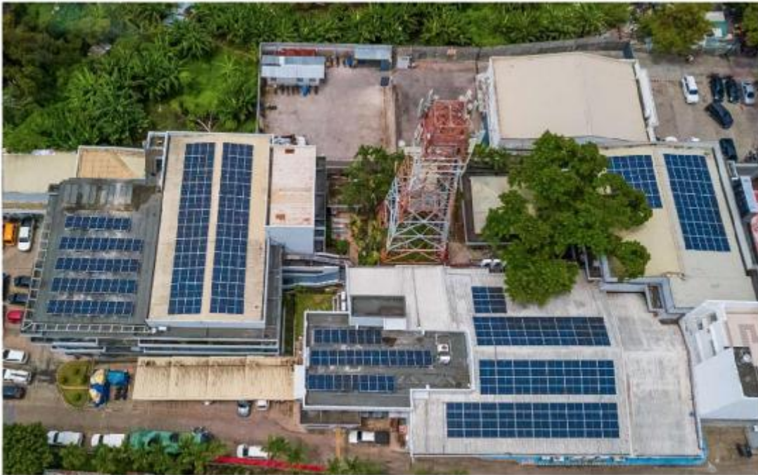
PHOTOGRAPH COURTESY OF PLDT | The PV panels will generate approximately 214,953 kilowatt hours (kWh) of solar power annually to augment electricity drawn from the commercial power grid, reducing PLDT's carbon footprint by 152 tons of carbon dioxide each year
