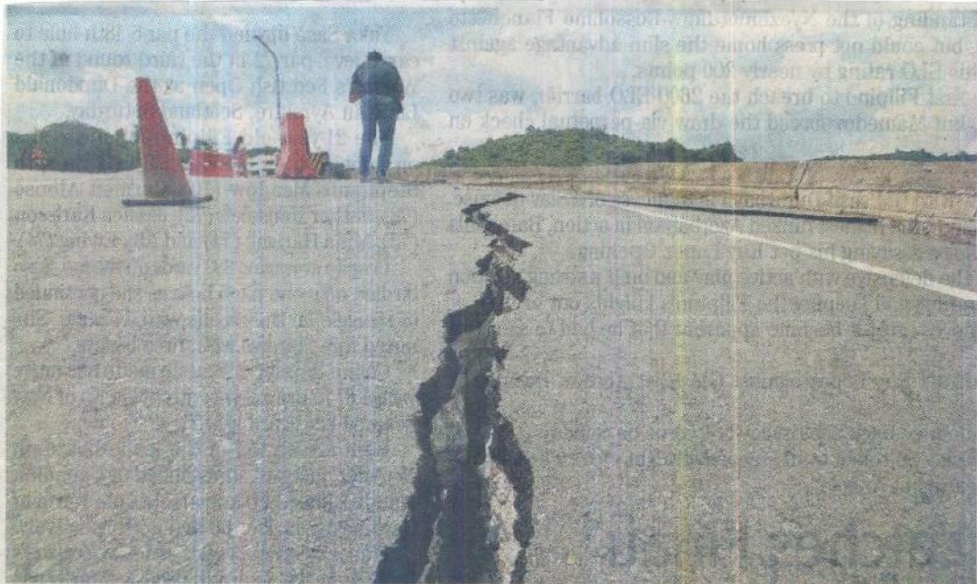
THE national road in Barangay Bio Lagangilang in Abra was damaged by a crack that runs across its length from the 27 July quake.
