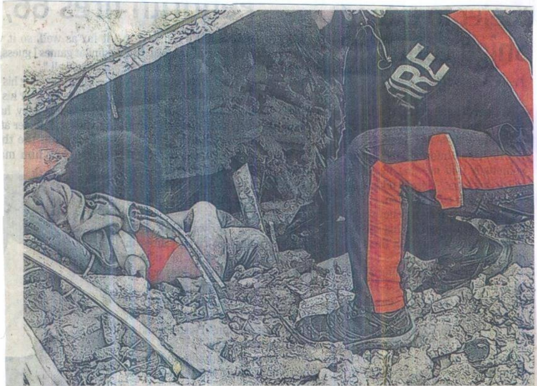
THIS building under construction in Buyagan, La Trinidad, Benguet collapsed and killed a construction worker during Wednesday morning's quake.
