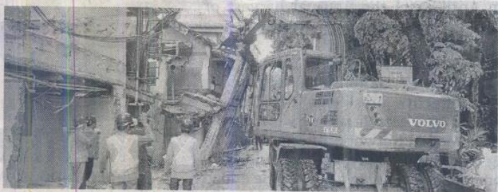
UNFINISHED BUSINESS In this photo taken on May 3, 2018, a week after the six-month closure of Boracay Island started, workers dismantle structures encroaching the road easement. Nearly four years later, the rehabilitation of the island is still unfinished. —NESTOR P. BURGOS JR.
