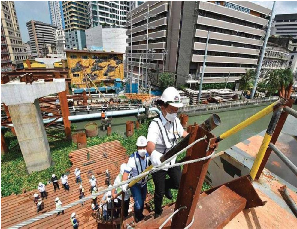
Public Works and Highways Secretary Roger 'Oging' Mercado inspects the ongoing China-donated Binondo-Intramuros Bridge project. PHOTO FROM DPWH WEBSITE
