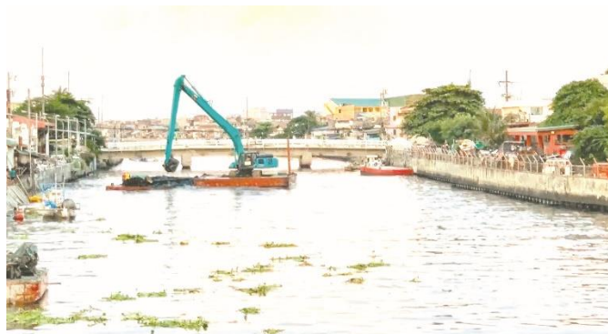
River dredging is one way of addressing flooding in prone areas. / Photograph courtesy of SMC
