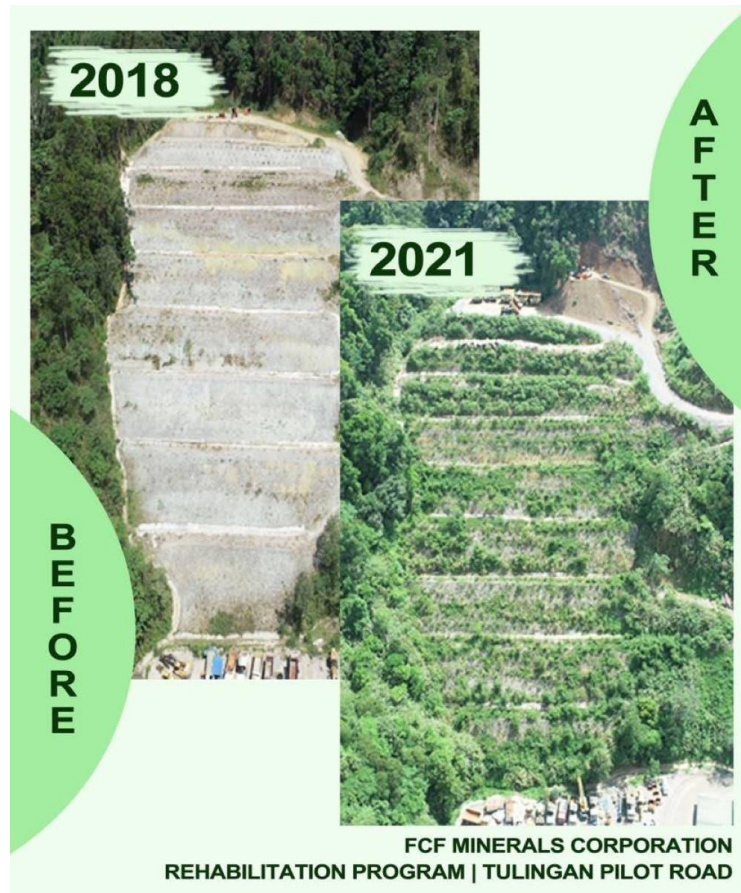
This photo combination shows the progress made by FCF Minerals in rehabilitating a road in Tulingan. CONTRIBUTED PHOTO
