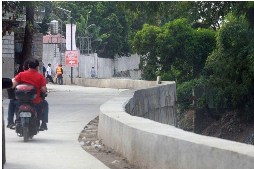
Photos shows the newly-constructed road in Zapote River Drive, Las Piñas City last October 29, 2018 Joven Cagande
