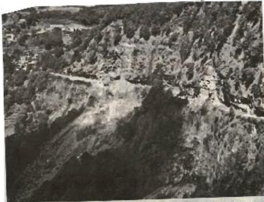
BLOCKED — A section of Mt. Uta Cliff in Bauko, Mt. Province is closed due to landslide caused by the Intensity 7 quake on July 27, 2022. (DPWH Cordillera Administrative Region)
