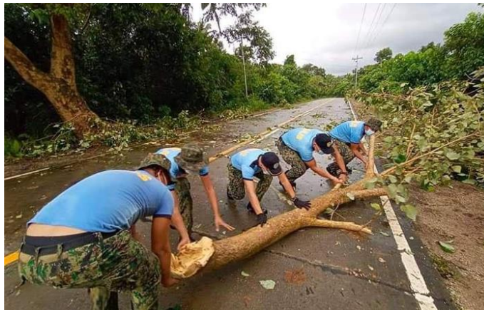
AFTERMATH. In Dinalungan, Aurora, authorities have a hard time and clearing the road of fallen trees. Aurora PPO
