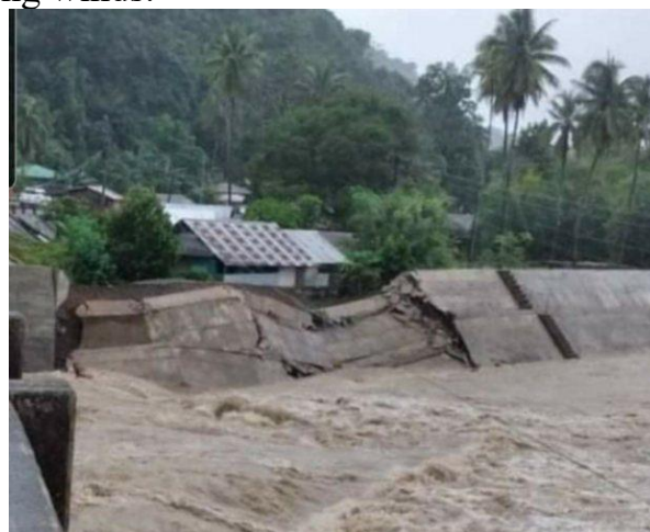
A portion of the Claver Baoy River dike collapsed due to the strong flow of floodwaters in Claver town. Photo from the Facebook page of the Public Information Agency – Surigao del Norte)
