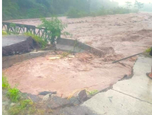
Part of the Budlingin Bridge in Alegria collapsed. (Photo from the Facebook page of the Philippine Information Agency – Surigao del Norte)
