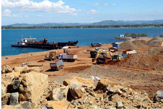
TRUCKS load rocks and soil containing nickel-ore minerals onto a barge in Sta. Cruz, Zambales, Feb. 8, 2017. — REUTERS
