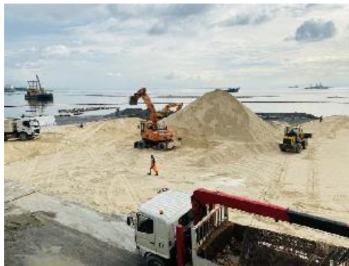
Engineering interventions are being done to ensure the white sand overlay will endure strong typhoon winds.
