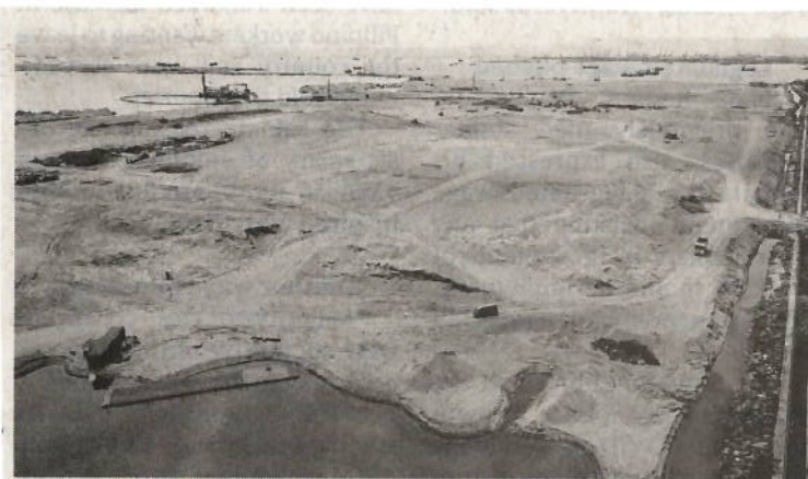
TAKING SHAPE Reclamation of this section of Manila Bay along J.W. Diokno Boulevard in Pasay City has been ongoing, as shown in this photo taken on June 25. Environmental advocates have expressed alarm over the impact of reclamation activities on Manila Bay's marine biodiversity. —GRIG C. MONTEGRANDE
