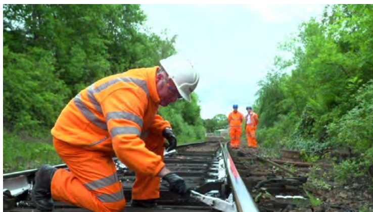
Train tracks are being painted white in some parts of the country to deflect the heat
