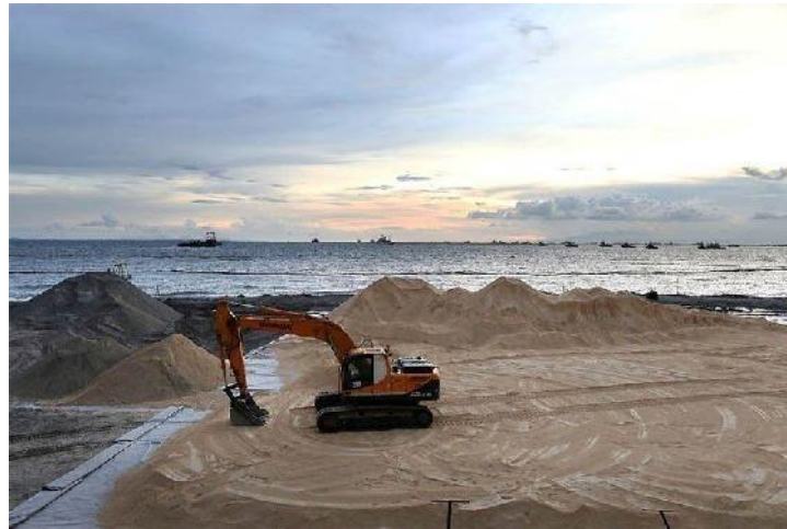
This undated photo shows the overlaying of crushed dolomites on the shore of Manila Bay. The STAR/Miguel de Guzman
