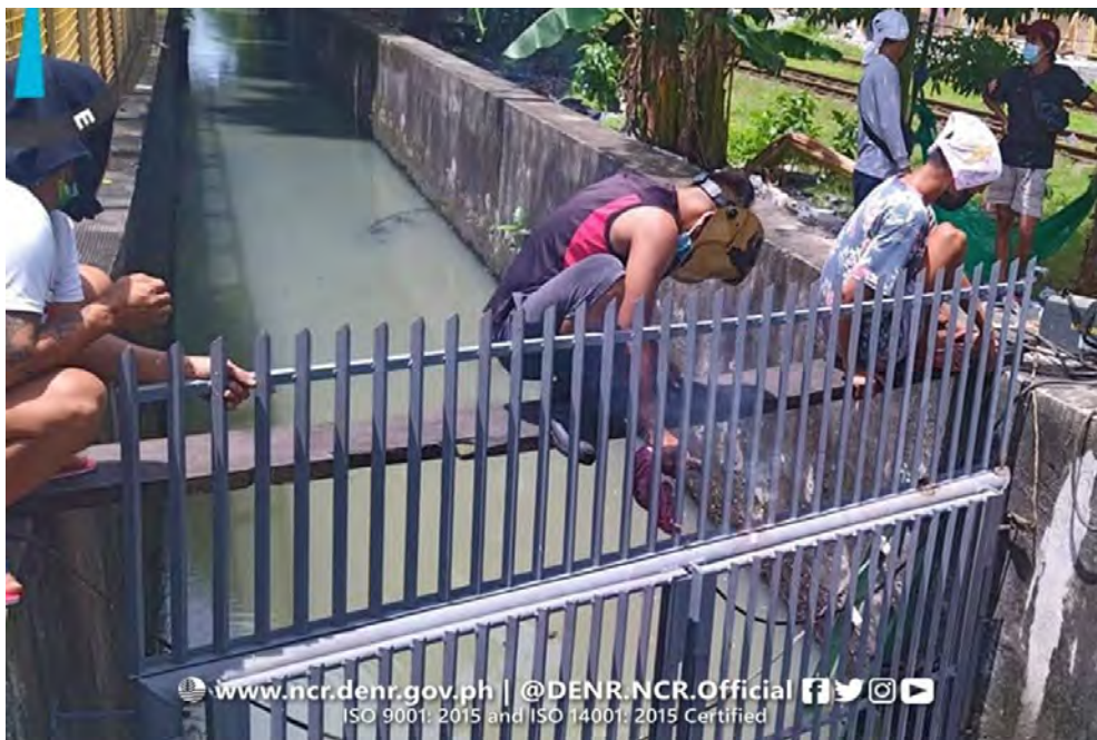
A trash trap being installed along Estero de Kabulusan in Old Antipolo Street, Barangay 356, Manila City. (PIA-NCR file photo)
