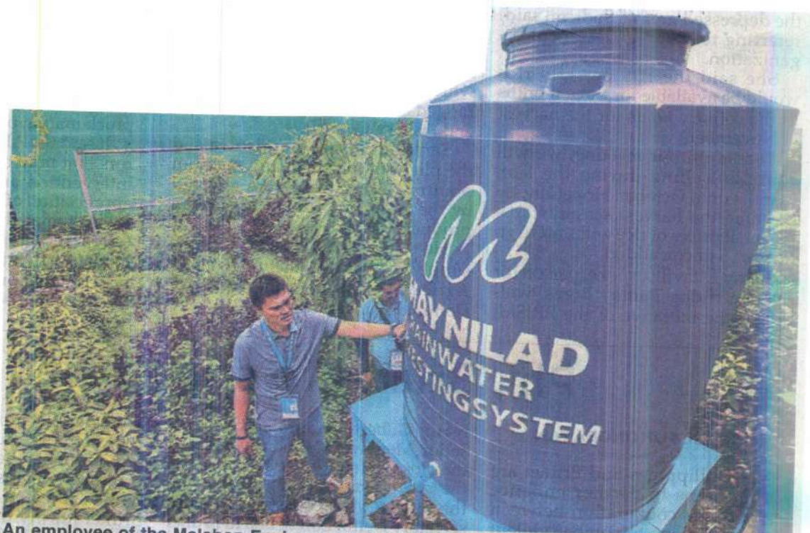
An employee of the Malabon Environmental and Natural Resources Office inspects the newly installed rainwater harvesting facility in Barangay Potrero yesterday. The DENR has called on local government units to establish alternative water sources as Angat Dam's operative level continues to drop.
