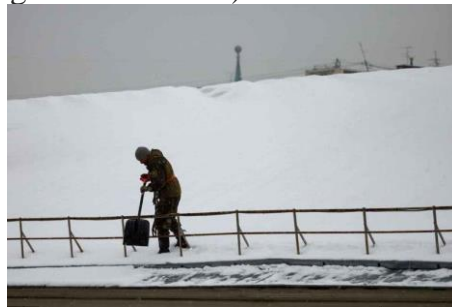
Moscow: A man removes snow from the roof of a building during a light snowfall in Moscow on February 11, 2021. Weather experts predicted record snowfalls in the Russian capital from Friday through to Sunday totalling up to around 40 centimetres (16 inches). AFP PHOTO
