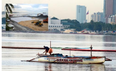
NEAR AND FAR. Workers continue to lay down the crushed dolomite used to whiten the beach at the Manila Baywalk (inset) while on the southern end of the bay near the Manila Yacht Club, a fisherman gets ready to set out for his daily catch on the waterway. Norman Cruz
