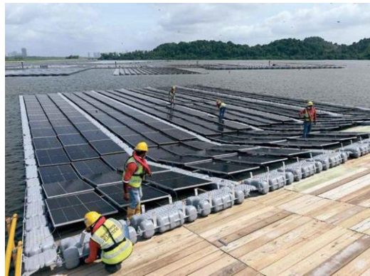
NEW FRONTIER This photograph taken on Feb. 3, 2021 shows workers assembling solar panels on the shore of the Tengoh reservoir as part of the construction of a floating solar power farm in Singapore. AFP PHOTO
