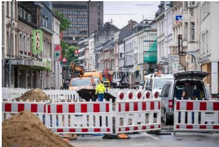
Clean-up and repair work continues on August 3, 2021 in Stolberg , western Germany, following the historic floods. AFP PHOTO
