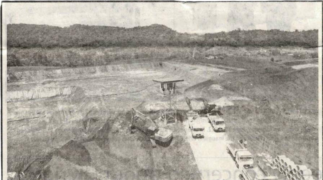
ENGINEERED SOLUTION The largest engineered sanitary landfill facility (SLF) in the country was inaugurated and commissioned on Tuesday, June 28, 2022, in Barangay Malimono, Marawi City and Barangay Kasayanan, Kapai, Lanao del Sur. The 31.7- hectare SLF would help address the solid waste management problem in the city as it can accommodate around 1 million tons of residual wastes. PHOTO FROM DENR
