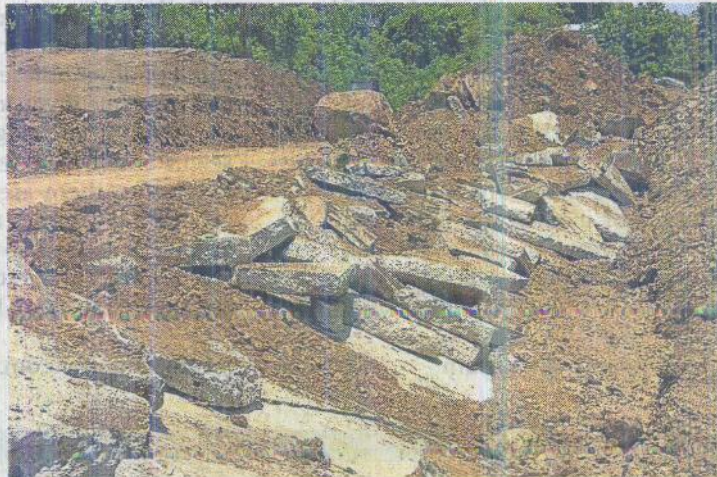
ERODED ROAD A large section of the bypass road at Sitio Corote in Barangay Upper Malagutay, Zamboanga City, crumbles when the ground underneath it was loosened by heavy rains that caused a landslide on Aug. 15. —JULIE ALIPALA
