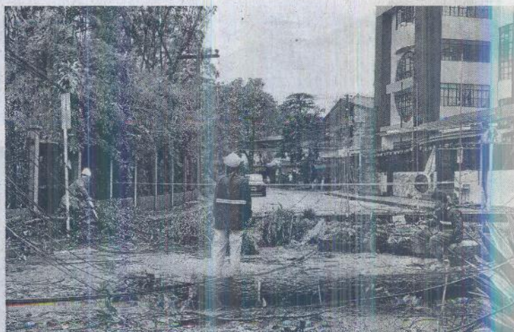
BAGUIO IMPACT Linemen of Benguet Electric Cooperative help clear a road and reconnect power lines on Thursday, a day after "Egay" also left serious damage in the summer capital.
