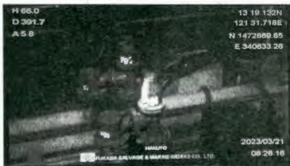
UNDERWATER photo taken by ROV Hakuyo show the leaking pipes, fittings and valves of the sunken MT Princess Empress around 395 meters below the surface of the sea in Naujan, Oriental Mindoro. PHILIPPINE COAST GUARD
