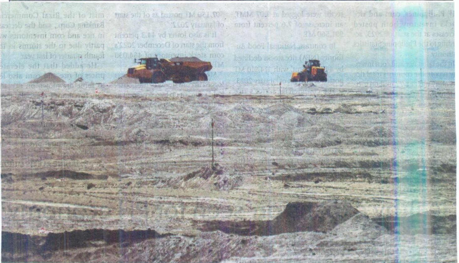
PUSHING THE SEA BACK Heavy machines flatten mounds of sand dumped by dredgers for use in a land reclamation project in Pasay City on Monday, April 3, 2023. PHOTO BY J. GERARD SEGUIA
