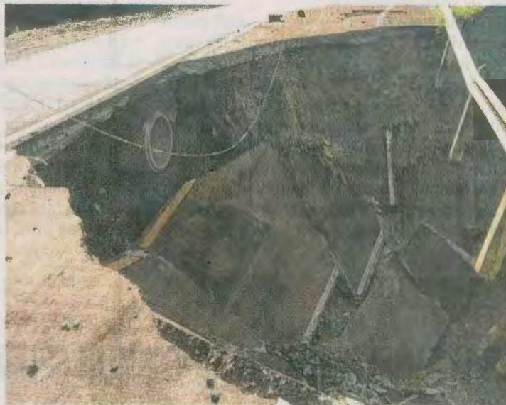
COLLAPSED ROAD A portion of the national highway that links the towns of New Bataan and Maragusan in Davao de Oro collapses after strong earthquakes rocked the province at dawn on Monday. —PHOTO COURTESY OF RUEBIL GARCIA
