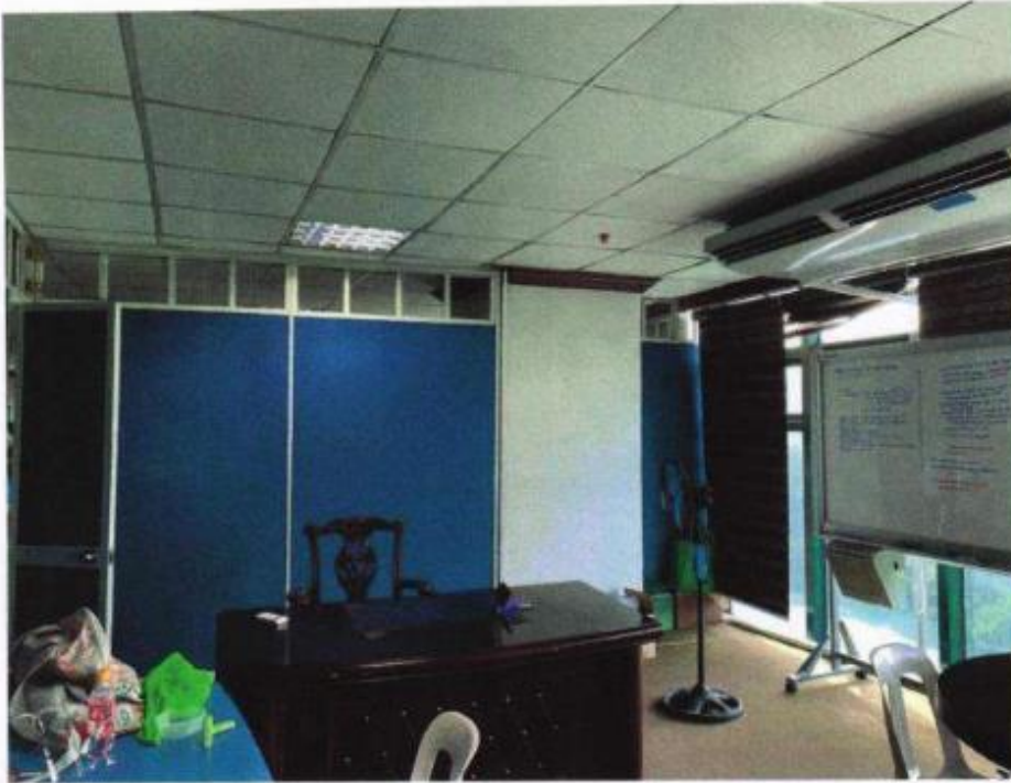
PIC 1: PHOTOGRAPH OF EXISTING INTERIOR OF THE OFFICE TAKEN AT THE RIGHT SIDE OF THE ROOM
